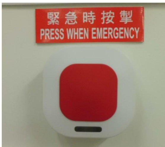
Emergency call button installed in B9W and B11W of Phase 2, HKSTP
