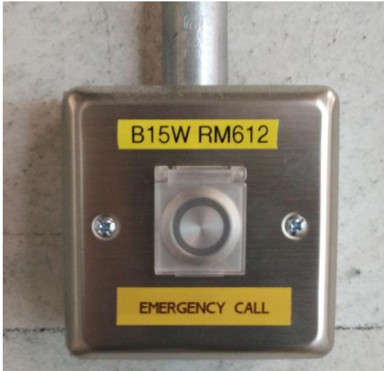
Emergency Call Button installed in Phase 3, HKSTP
