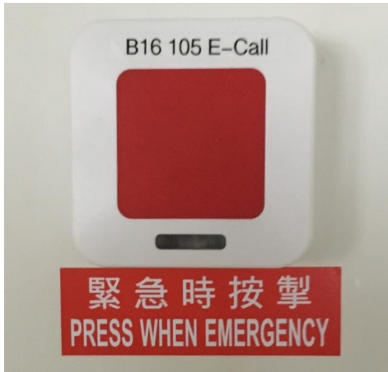
Emergency call button installed in B8W and B10W of Phase 2, HKSTP
